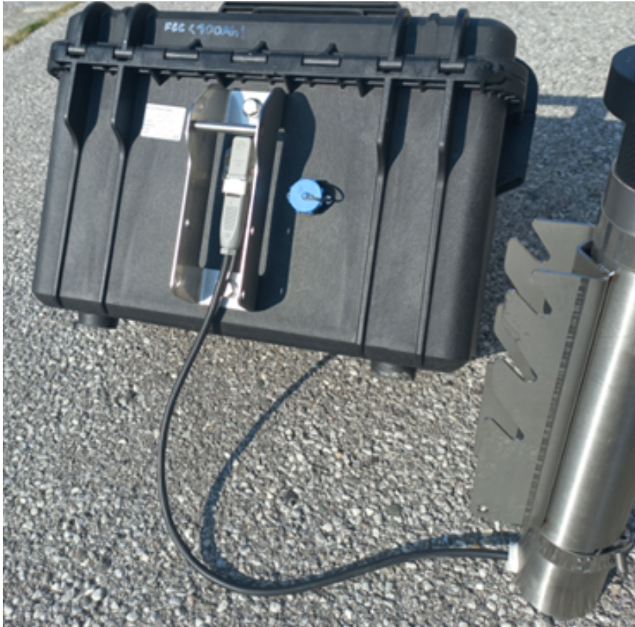
Connection at the battery box (article 100507).
